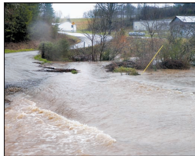
Roadwork continues on Lowe's Mill, which was washed out during torrential rains on Jan. 30th. Photo/Todd Forrest
