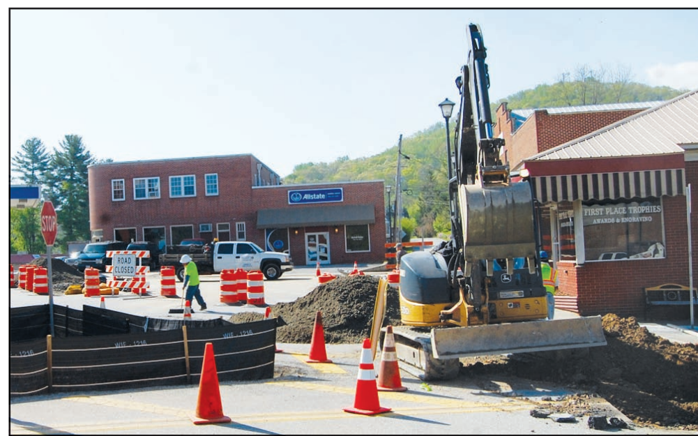
The Downtown Streetscape project is progressing on schedule according to Mayor Jim Conley. Photo/Lowell Nicholson
