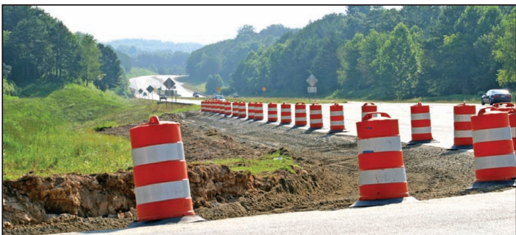
The County Road Department is reworking the turning lane on GA 515 leading into Walmart.
