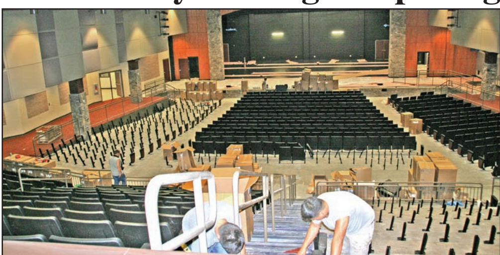
Workers put the finishing touches on the auditorium at the new Fine Arts Center. Photo/Shawn Jarrard
